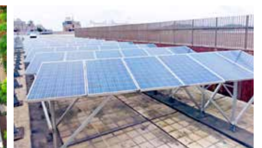
▲ Taipei-Solar Power Generation System
